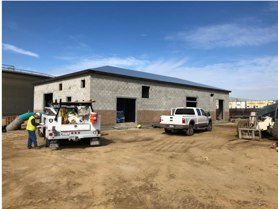
Industrial Tank 13/Pump Station
