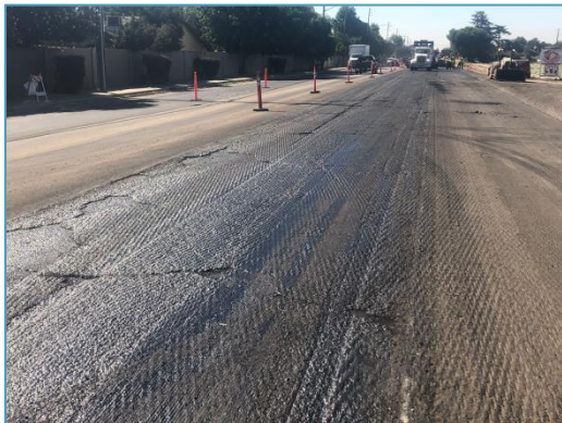
Surface Condition Prior to Leveling
