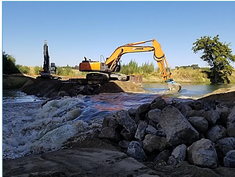
Contractor removing the cofferdam that was used to divert the Tuolumne River
