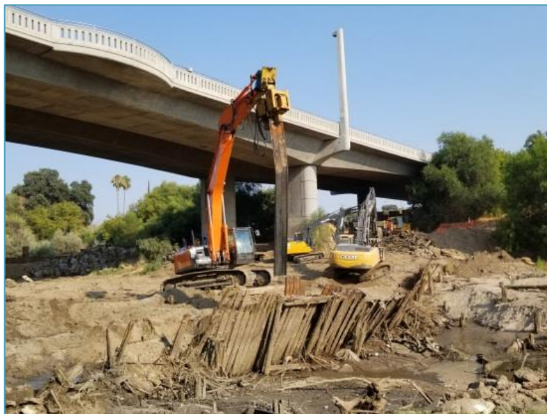
Contractor removing twenty foot long sheet piles from remnant Dennett Dam structure.
