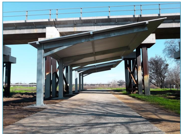
Union Pacific Railroad Pedestrian protective covers installed to protect trail users crossing underneath the railroad from falling debris.
