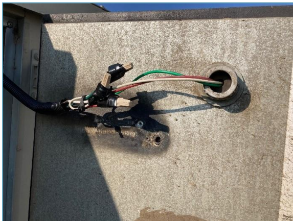
Wire arc damage due to faulty connector and/or moisture intrusion
