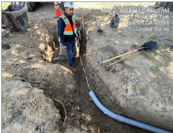
Mule tape placement AT&T conduit in joint trench at Colorado Avenue and Garden Avenue
