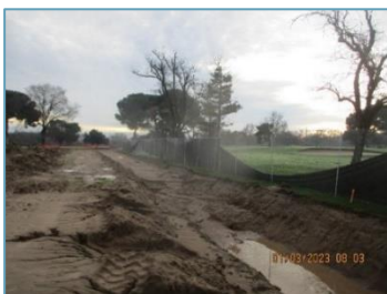
Site conditions after storm
