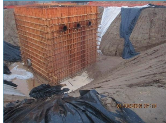
Flooding at pump station due to storms
