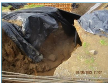
Erosion due to storms
