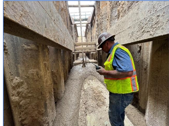
60-in. Fiberglass Reinforced Polymer Mortar Pipe native slurry trench backfill operations along Garden Avenue
