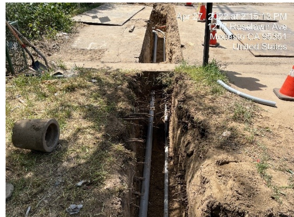
MID and AT&T joint trench reroute at Colorado Avenue and Garden Avenue
