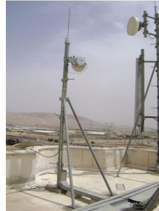
Point-to-Point Wireless Antennae
